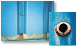
Loss of pull over value on the fastener head and unsightly rust stains due to corrosion of fastener
