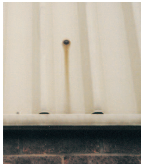
Atmospheric pollution can lead to corrosion of the fasteners.
