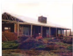
Adverse effect of coastal salt air on carbon fasteners in post-frame construction
